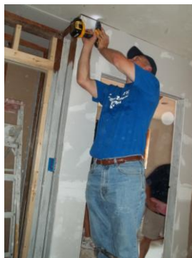
Left: Robert Woudstra (left), President & CEO of Farmers Insurance Group, and Mike Foley (right), CEO of Zurich North America, work with friends and co-workers to install insulation at the Bayou District Foundation's house on Harrison Avenue, while in town for the Zurich Classic in April.
