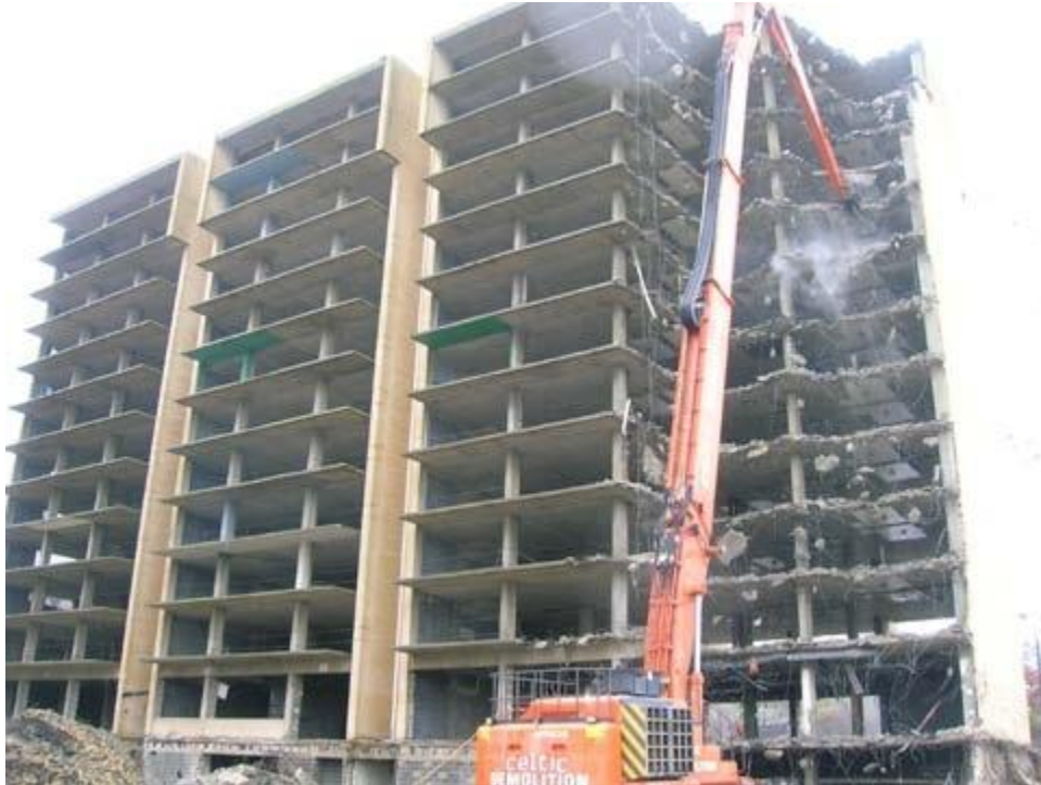
Above: D.C.'s old Capitol Gateway housing project during demolition in 2005 (DC Housing Enterprises) . Below: Capitol Gateway today. (Henson Development) .
